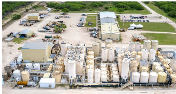
Alta Mesa Central Processing Plant, Texas, USA
